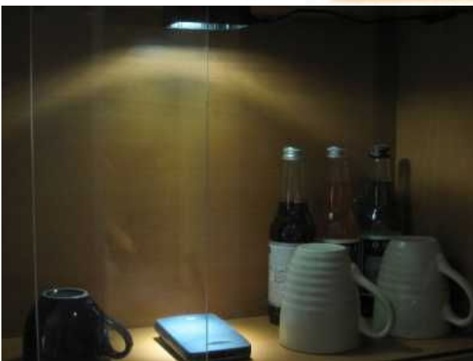
LLK-03 LED Lighting/Meter Heatsink Plate Kit mounted with various LED arrays and meters.
