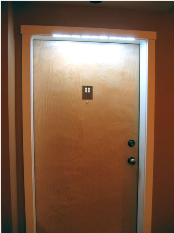
Door entrance lighting.
